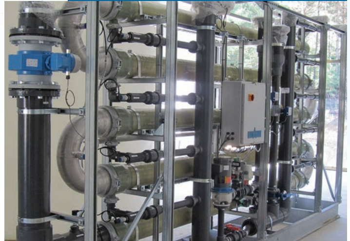
Ultra Filtration Skid
