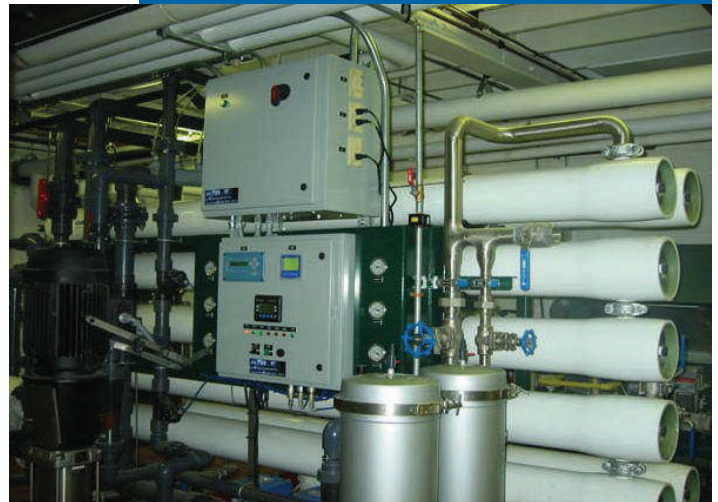
Reverse Osmosis System
